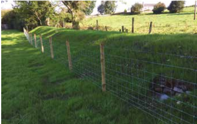
Earth bund to temporarily store runoff during storm events at Greysouthern. A 150 mm pipe through the bund allows the field to drain down after flood events. With thanks to landowner and Greysouthern Parish Council. Image © Cumbria County Council.
