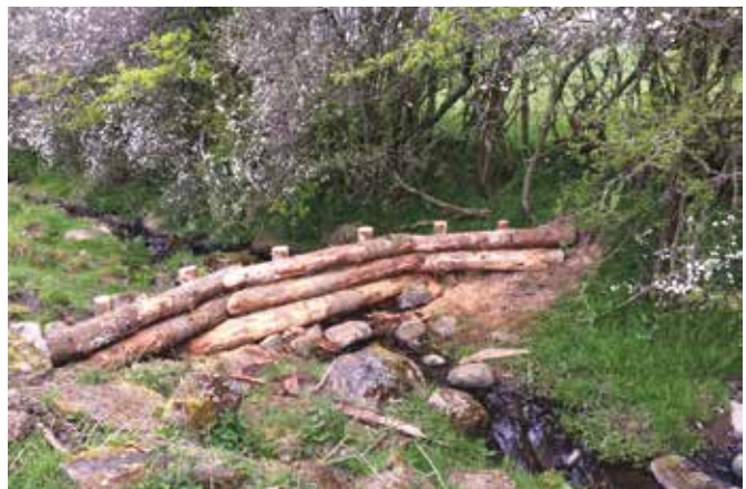
Leaky barriers on Dovenby beck, near Cockermouth © West Cumbria Rivers Trust
