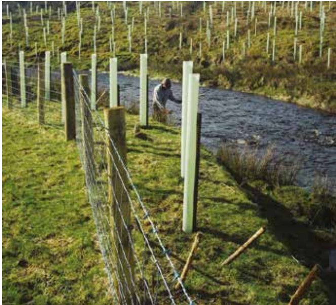
Bankside fencing and tree planting on Cam beck, River Ribble. © Woodland Trust.
