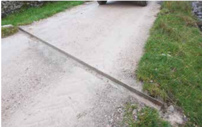
Cross drain to divert run-off from a farm track. © West Cumbria Rivers Trust.
