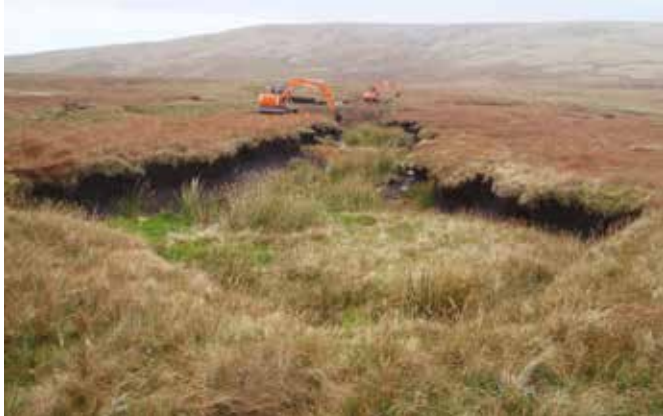
Regrading the steep bank of a peat hag on an area of degraded peat on Kinmont Buckbarrow, near Millom, Cumbria. © Cumbria Wildlife Trust.
