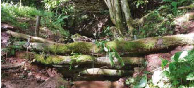
A series of 24 woody dams installed in Cumrew beck to reduce flooding in Cumrew village, near Carlisle. © Eden Rivers Trust
