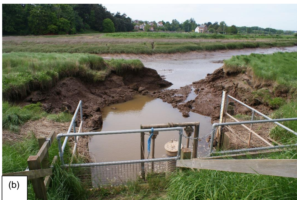
Figure 5.3 Regulated tidal exchange scheme at Goosemoor: (a) sluice structure facing into the estuary and (b) culvert and stop logs inside the site
