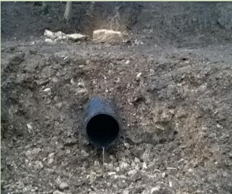
Photo 6: Culvert and soakaway, Ebworth Estate, January 2015 (source: Chris Uttley, Stroud District Council)
