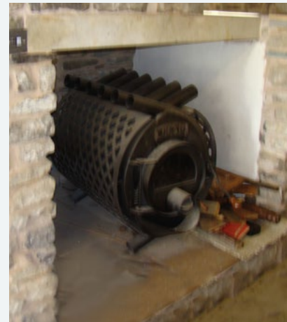
Figure 5 Wood-burning stove, housed within body of stone staircase (German 18kw design)
