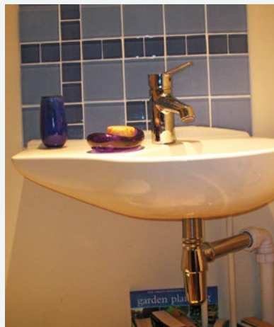
Figure 8 Downstairs sink – no vanity unit
