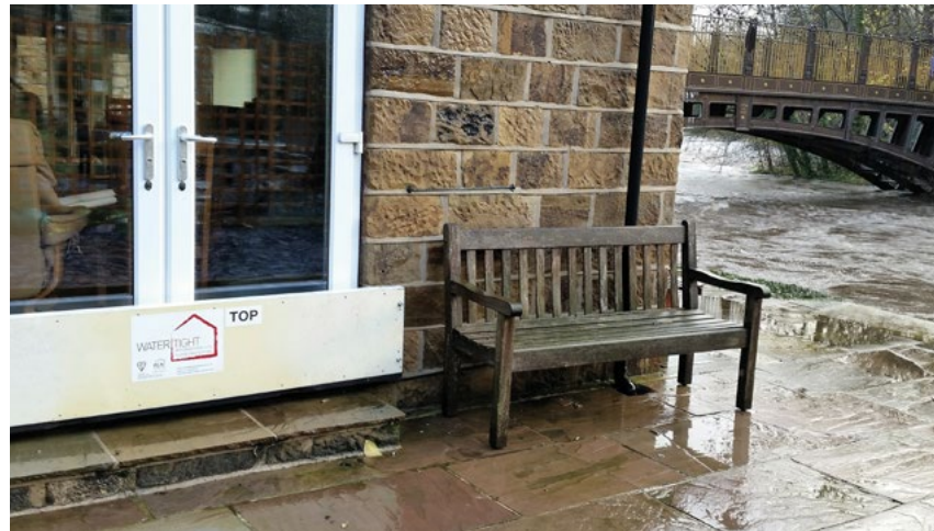
Figure 2 Although barriers were in place, the river had an unpleasant surprise in store
