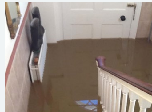
Figure 1 Hallway during 2015 flood
