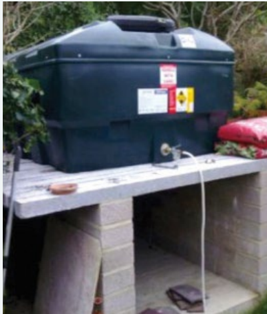
Figure 3 Fuel oil tank on raised plinth
