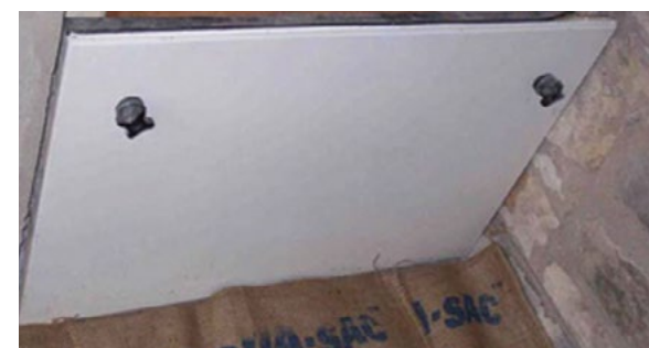
Figure 3 Door guard fitted to the internal doorway
