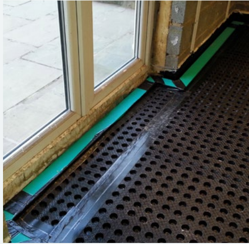
Figure 5 Channels and membranes with sumps and pumps to remove water
