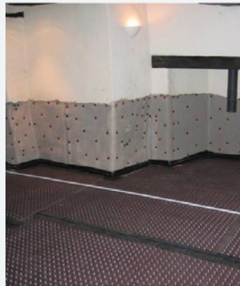
Figure 3 Internal walls now covered with a mesh membrane, and floors are covered with a studded membrane
