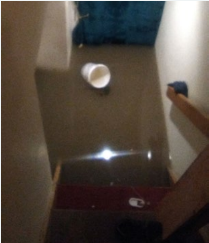
Figure 1 Hallway pictured from original stairs during the flood
