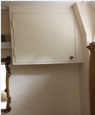
Figure 7 Unobtrusive cupboard to house meters
