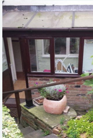
Figure 4 Kitchen and utility room are 6" lower than rest of house
