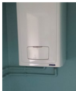
Figure 3 Boiler supplying CH & hot water has been moved upstairs
