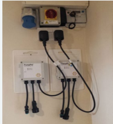
Figure 1 Sump pump controls are on separate circuit, fixed high above water level
