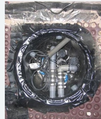
Figure 4 Two sumps (similar in size to a domestic dustbin) contain pumps designed to operate at different water depths.
