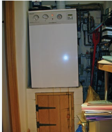
Figure 4 Boiler on plinth
