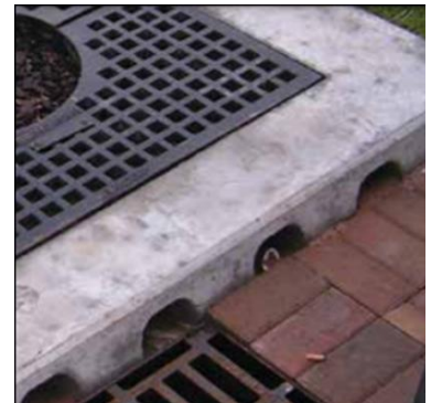
Outlets blocked by other features
