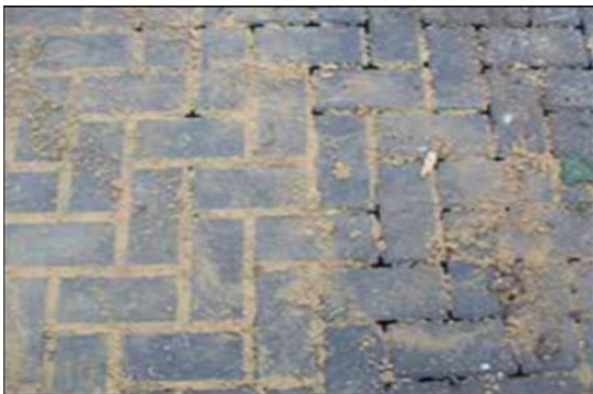
Blocked permeable paving
