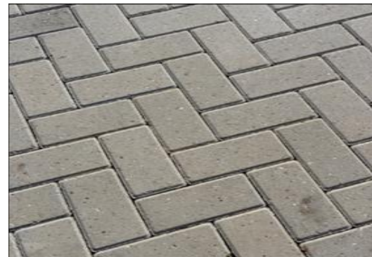
Author's photo of so-called 'permeable paving' which isn't permeable at all; there are no notches in the pavers or gaps between them
