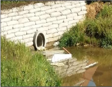
Rubbish could create blockages
