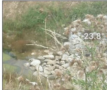
A collapsed structure creates a blockage that prevents water from leaving the feature
