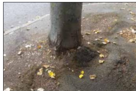
Tarmac around a tree whose roots are pushing up the surface of the pavement.
