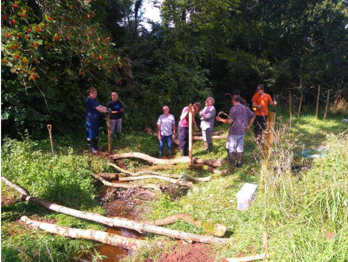
Photo 1: Apprentices from the Roe Catchment Community Water Management Group and Eden Rivers Trust installing leaky dams, August 2016
