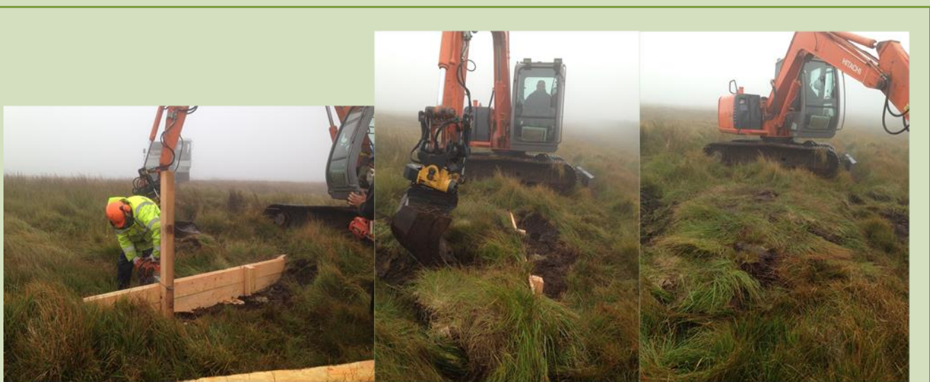
Photo 2: Construction of wooden block used to block drainage ditch, November 2014 (source: Exmoor Mires Partnership)
