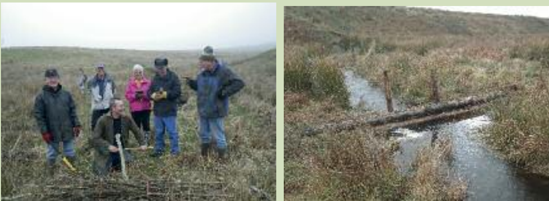
Photo 3: Volunteers working as a team (left) to produce brash bundles to add to the timber sluice constructions (right). Brash material was acquired from Environment Agency tree maintenance work further down the catchment and transported to site by a project partner (source: Newson and Gibson 2015)
