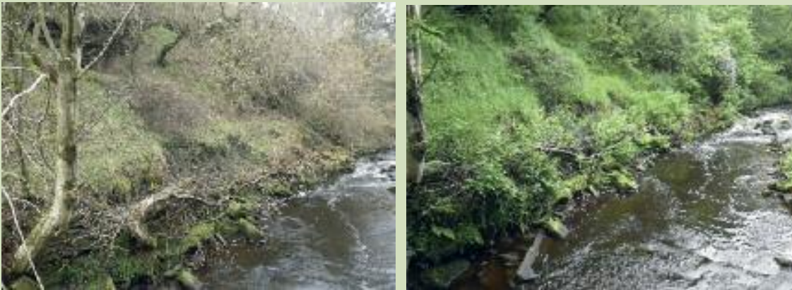
Photo 3: Left: A living tree is laid to reduce river bank collapse at old quarry/mine site. An additional trunk is secured on the river bed to direct flow away from eroding bank. Right: One season of growth demonstrates how well the bank is repairing. This is a fixed point photography site (from marked post on footbridge) (source Newson and Gibson 2015)
